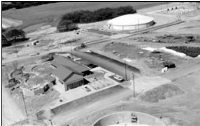
This shot of the ASR under construction in March shows just part of the large site. Much of the mechanical structure, and all of the storage, is underground.
