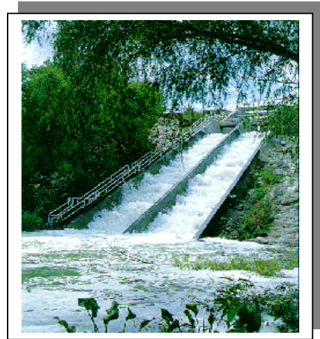
Dos Rios Treatment Plant
