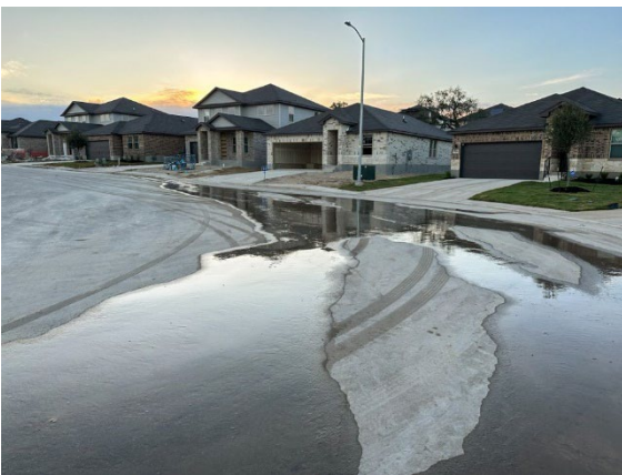
Water run-off from improperly working irrigation system pools in the street. This amounts to water waste under SAWS' Conservation rules.
